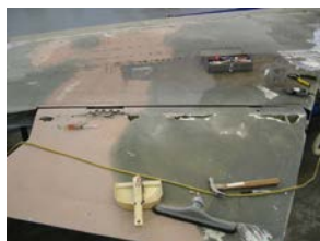
Flap corrosion and damage.
