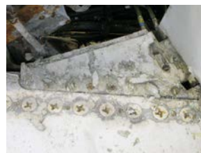
Wing panel corrosion.
